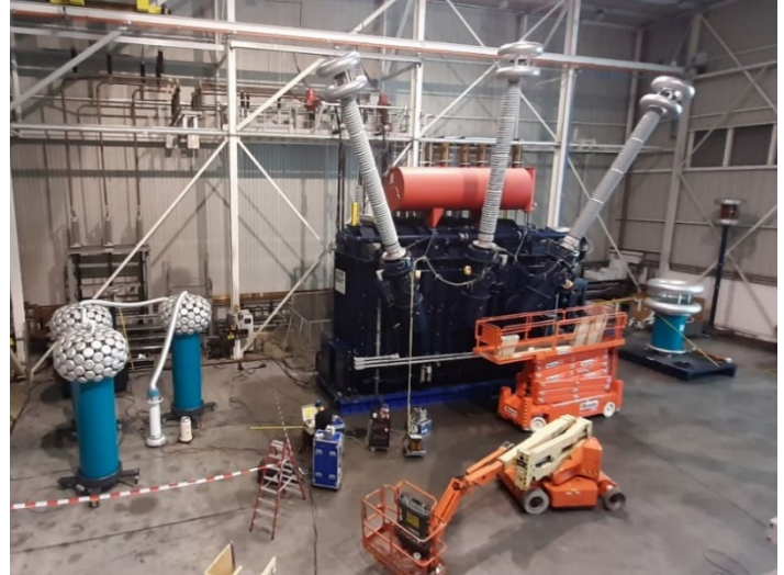
Testing of a transformer at Royal Smit Transformers
